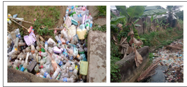
Figure 1. PET/PS blocked drains.
