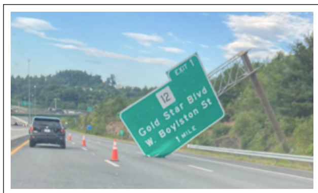
Figure 1. Collapsed sign support.
