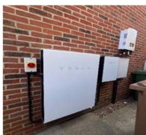
Fig. 6. Tesla Powerwall battery and solar inverter installed at Seymour Road project. 41 Seymour Road.
